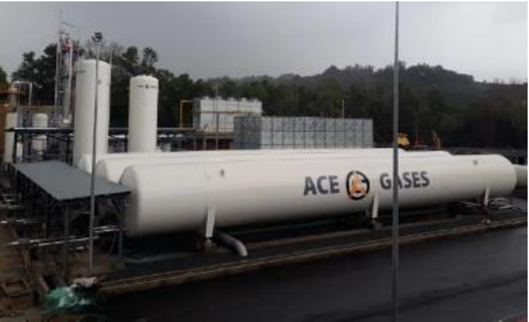
LCO2 Plant 1 (commenced 4Q 2019)
