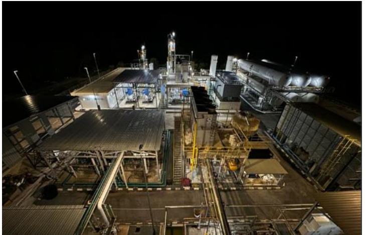
LCO2 Plant 2 (commenced 1Q 2024)
