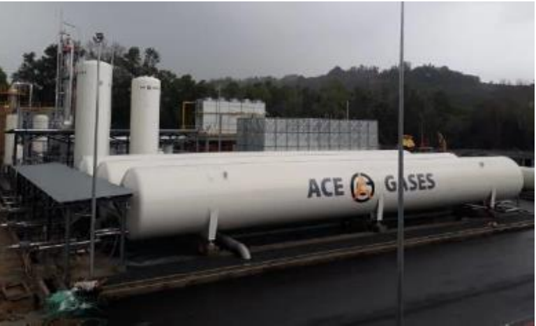
LCO2 Plant 1 (commenced 4Q 2019)
