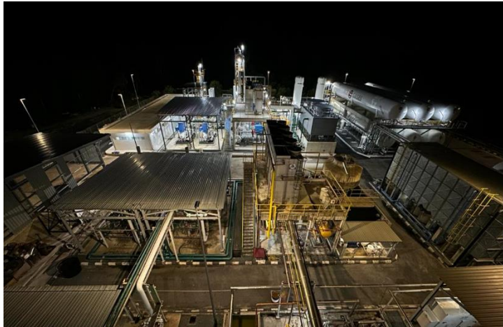
LCO2 Plant 2 (commenced 1Q 2024)
