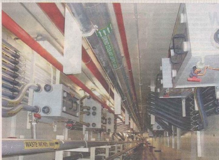
Kelington assembles and installs 'ultra high purity' pipes for use in industries.
